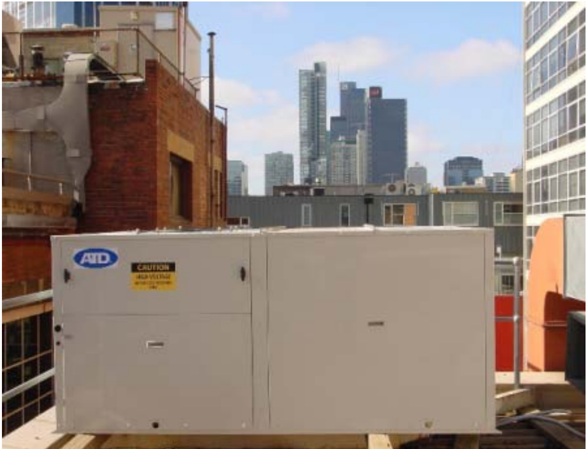
HVAC Packaged Rooftop Air to Air chiller (model: LAAHCP30) replacement to a Bank of China in Melbourne
